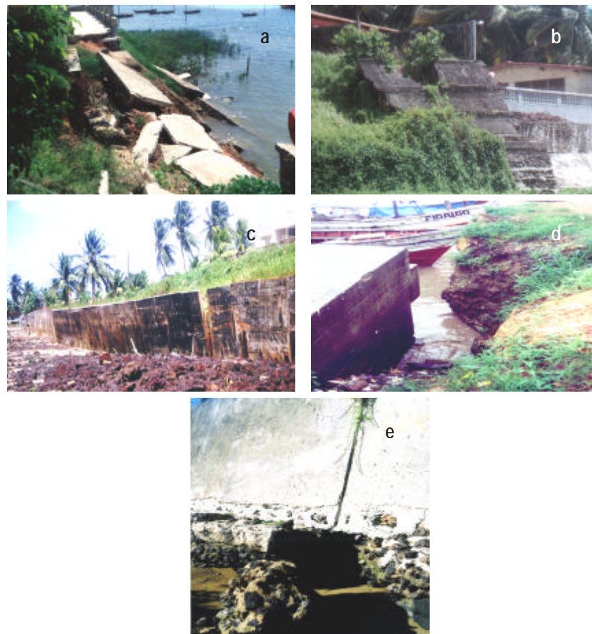
Figure 4.4 Principal types of structural problems found in protection works, (a) rupture; (b) collapse; (c) inclination; (d) back erosion and (e) basal erosion.
