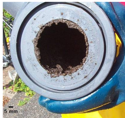
Fig. 103. Biofilm and solid attachments on the internal wall of the 63 mm in diameter outlet pipe from the biofilter (nitrification) tank. The sludge is approximately between 3 mm and 6 mm thick. The photography was taken on day t_{435} .
