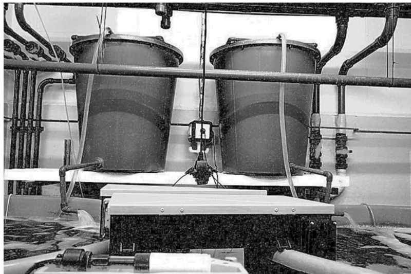
Fig. 13. Side view of the two additional external trickling biofilter (one for each tank), installed during days t_{239} and t_{431} of the study period.
