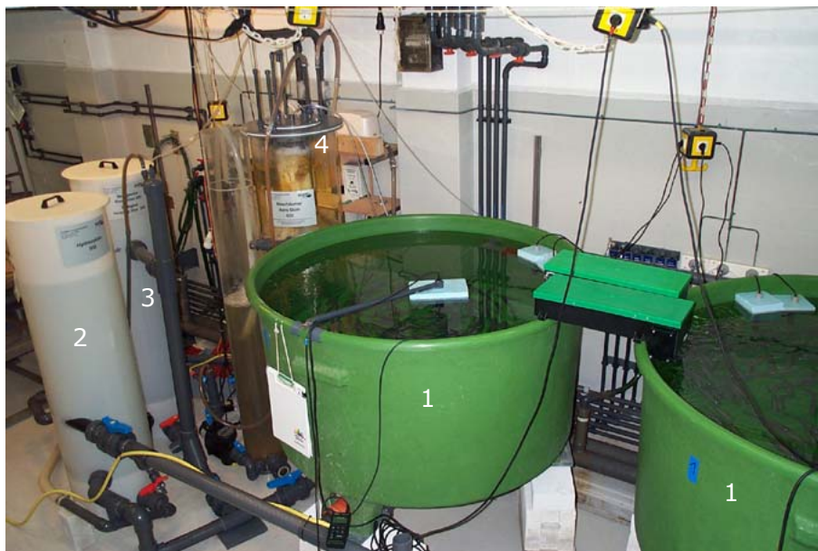
Fig. 2. The closed marine recirculating aquaculture system (RAS) consisting of the following essential components: (1) fish tanks, (2) swirl separator, (3) biofilter and, (4) foam fractionator.
