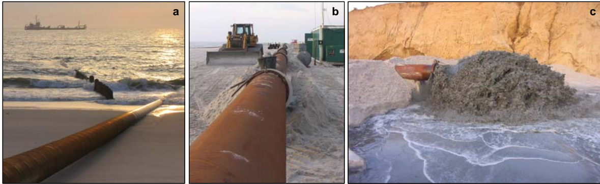
Fig. 3.14: Sand replenishment at the west shore of Sylt. The sand gets transported by ship to the shore (a), and washed through pipelines to the beach, where it gets distributed by bulldozers (b and c).
