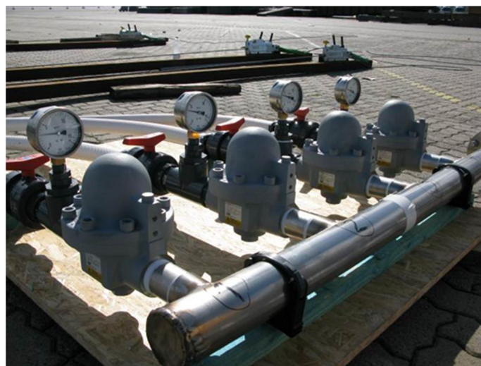
Fig. 6-5 Pressure adjusting valves, manometers and flow valves for adjusting air flow rate and overpressure.
