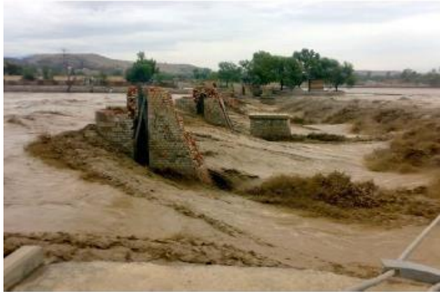
Figure 42:Washed-out Munda Headwork due to Flood Water (source: NDMA 2016)
