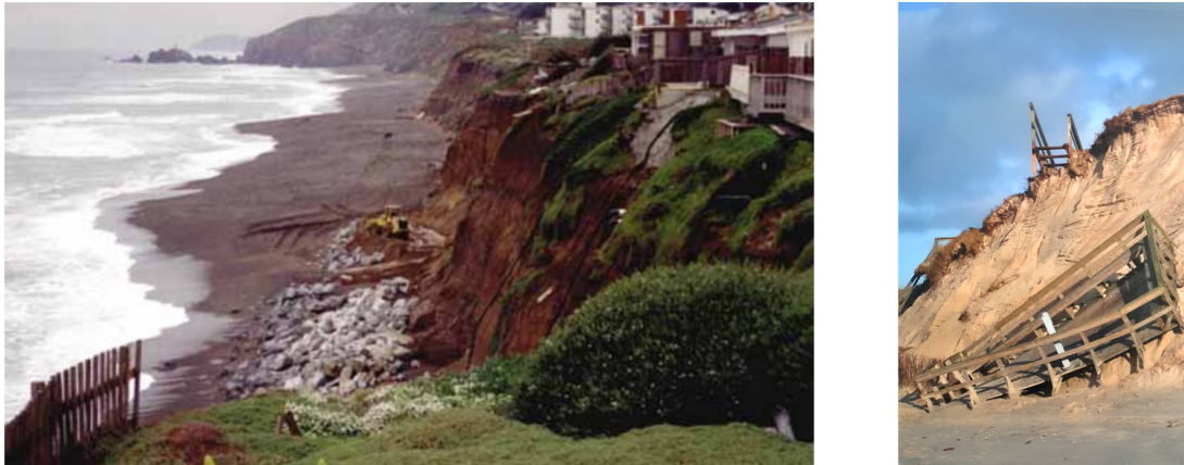
Figure 1.1: Left: Northward view along the approximately 30-m tall sea cliff at North Explanade beach in Pacifica, California in 1997. Source: U.S. Geological Survey, http://pubs.usgs.gov/pp/pp1693 . Right: Visitors platform damaged by erosion of the dune face at the Southwest coast of the island Sylt, Germany in 2015. Credit: Jochen Horstmann.
