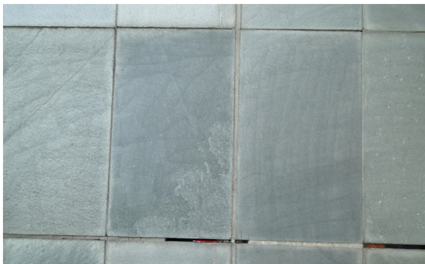
Figure 8. Phyllitic Quartzite facade panels (transverse length = 50 cm) (almost 60 years old); Alta Quartzite/Norway.
