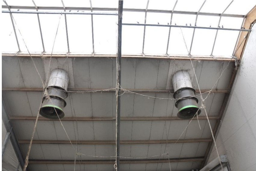
Figure 14 View of the two ventilators inside the units.
